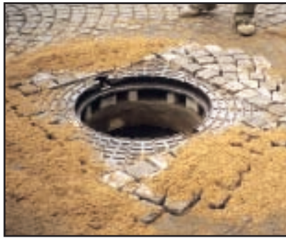
A manhole cover designed to match perfectly into its environment.
