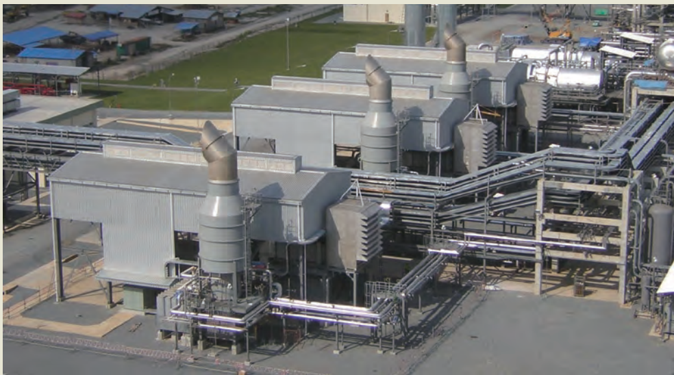
H-25 Gas Turbine Project (Indonesia)
