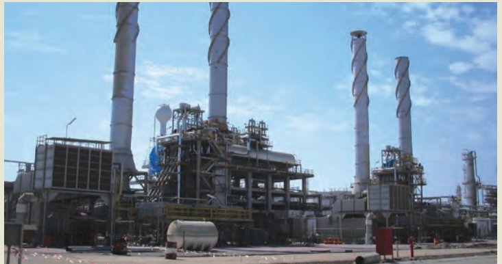
H-25 Gas Turbine Cogeneration Plant (Oman)
