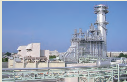
H-25 Gas Turbine Combined Cycle Plant (Japan)
